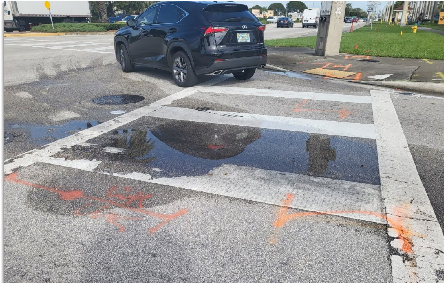
Detail of faded markings and pavement distress
