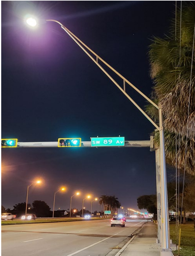
FDOT Aluminum Pole installed with LED luminaire
